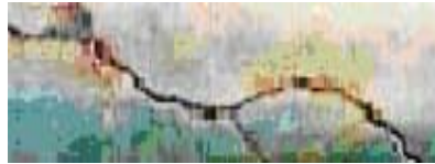
Fig. 9 Stress corrosion cracking.
